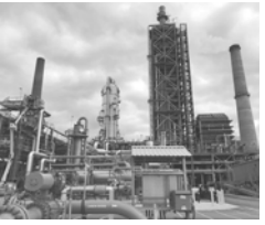
Equipment used to capture carbon dioxide emissions at a coal-fired power plant in Thompsons, Texas. REUTERS
